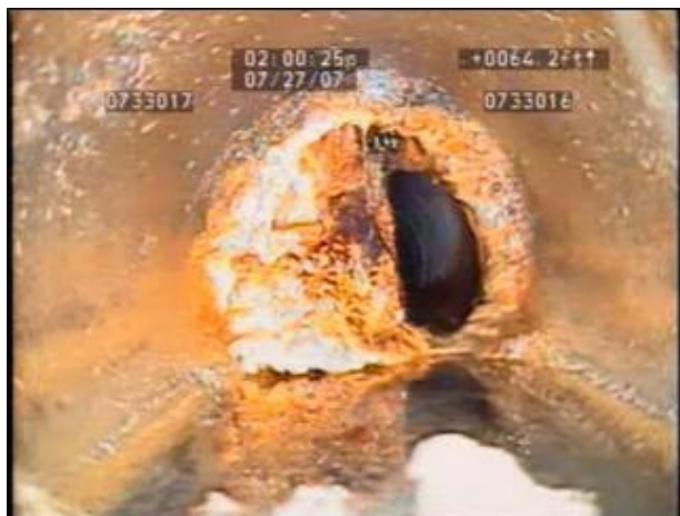
Example of a sewer severely plugged by grease
